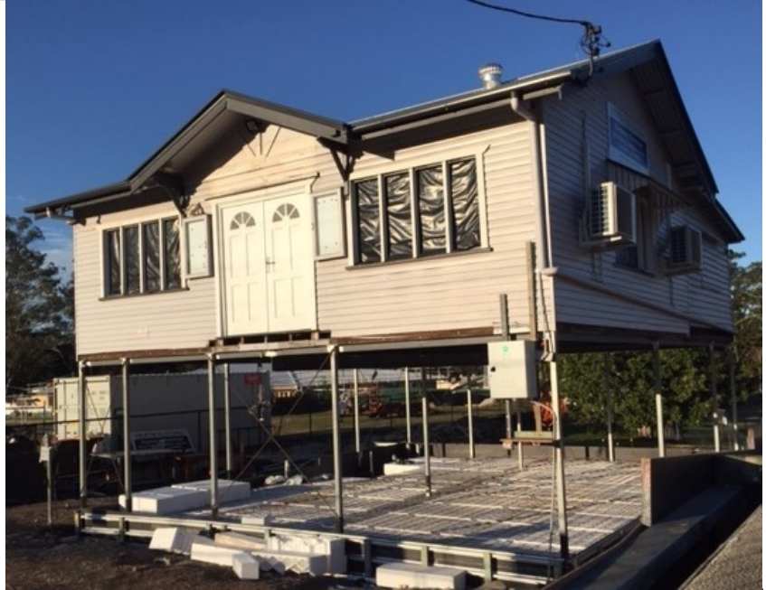
It's high and dry! Our Fulcher Road premises are raised and ready for a concrete slab to be poured downstairs to provide a practical flood-free work space. The rotting timber posts have been replaced by shiny steel ones, and the upstairs work area is supported by some solid steel beams.
